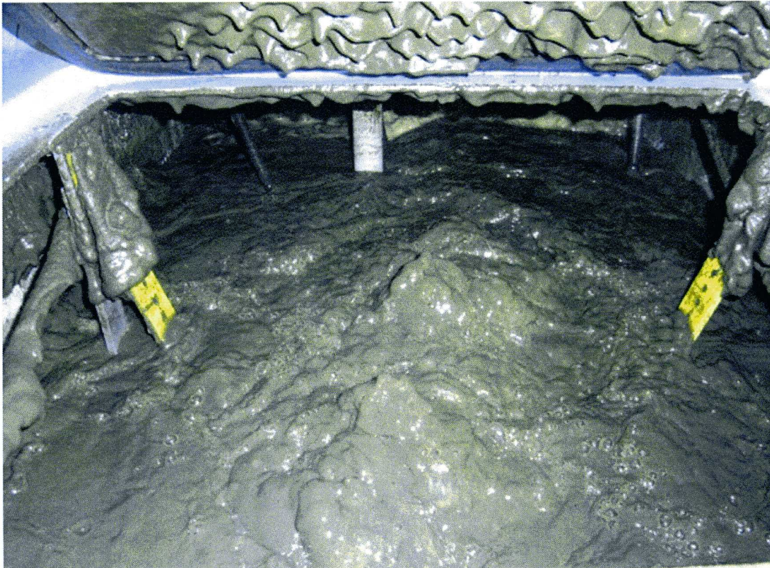
Figure 6: View into membrane-bioreactor in operation
