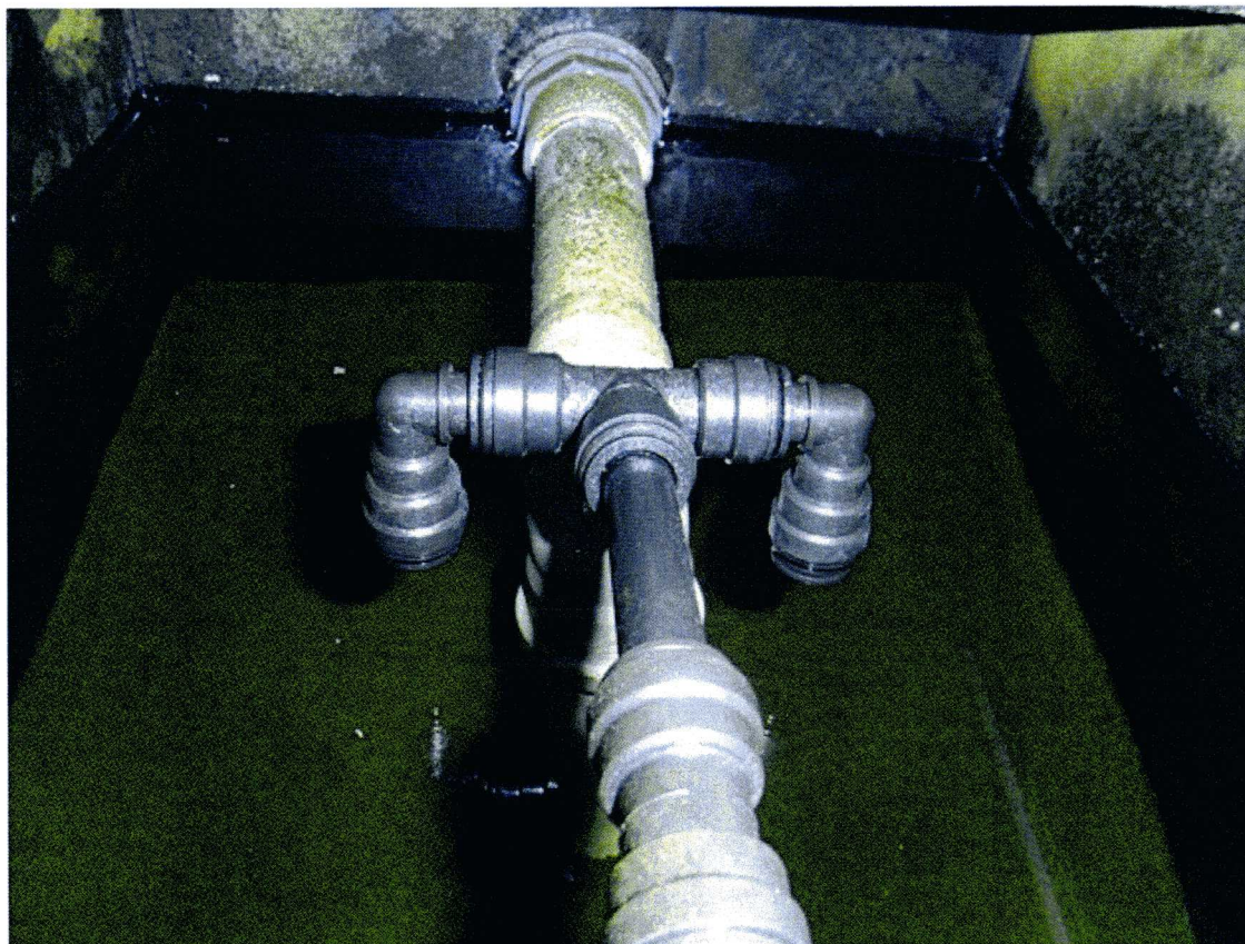
Figure 7: View into the first P-Module in operation
