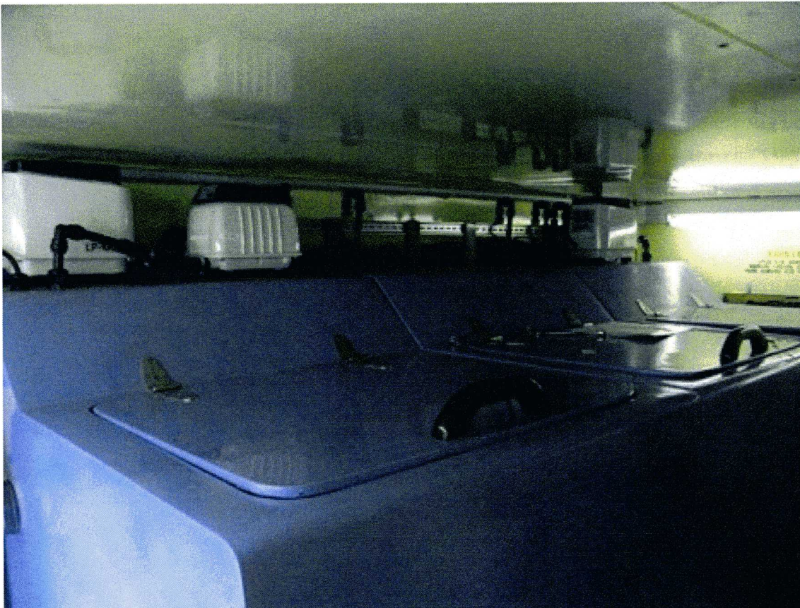
Figure 2: Picture of the treatment plant (3 GRP-tanks) in the test-container
