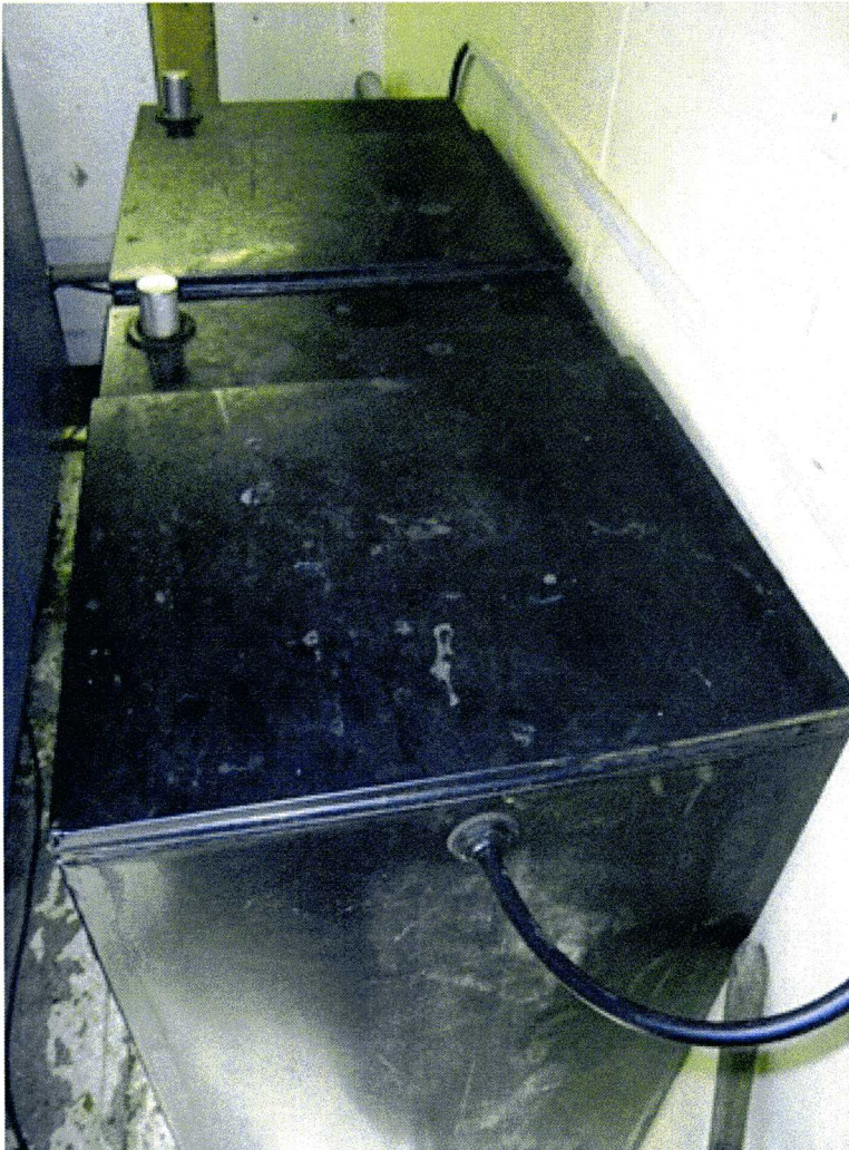
Figure 3: View on the P-Elimination section (PE-tanks)
