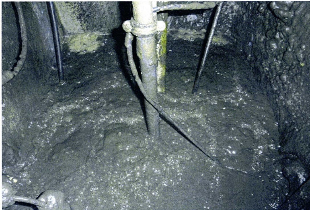
Figure 5: View into the biological chamber of the plant
